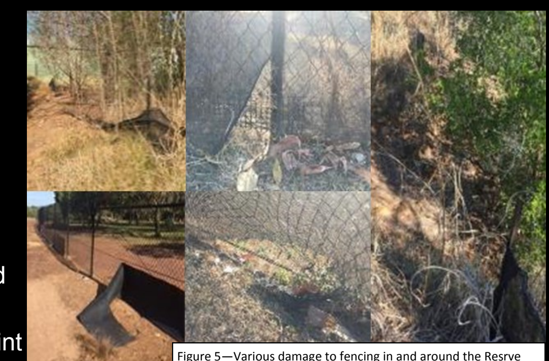
Figure 5—Various damage to fencing in and around the Reserve
